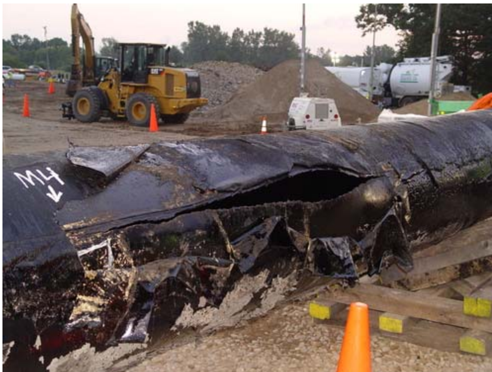
Ruptured Section of Pipeline 6B (Photo from National Transportation Safety Board)
